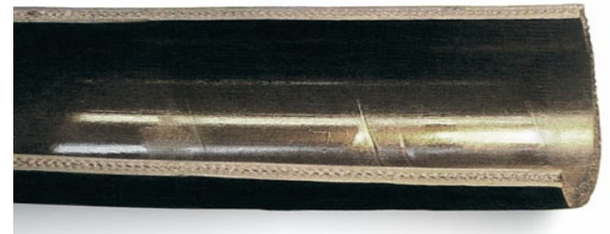
Visible seams in the lining
